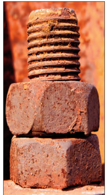
Red rust makes removal of nuts difficult at best.
