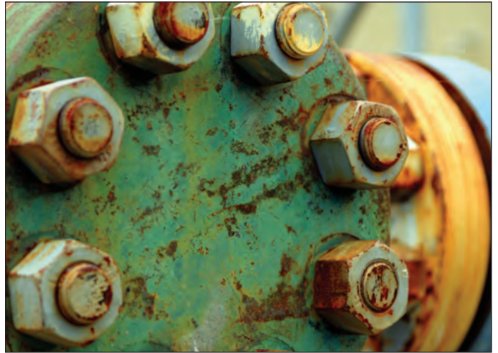
Large bolts and washers become corroded when conventional marine paints are used.
