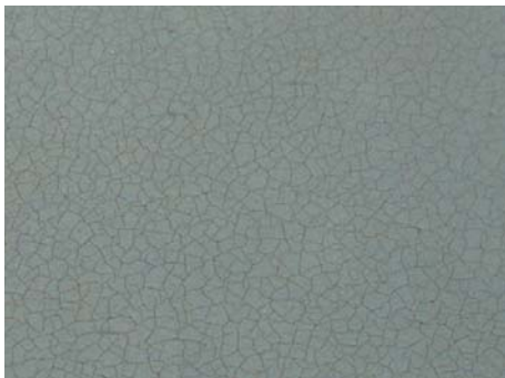
"Mud-cracking" caused by the application of too much coating.
